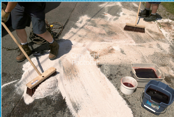
Non-hazardous OCFEC Internal Oil Spill Clean Up
